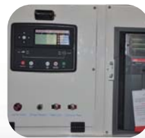
Control Panel & MCB
